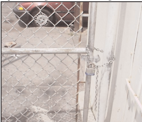
Blocked exit paths and locked exit discharges
